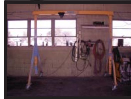
Gantry A Frame with Hoist
